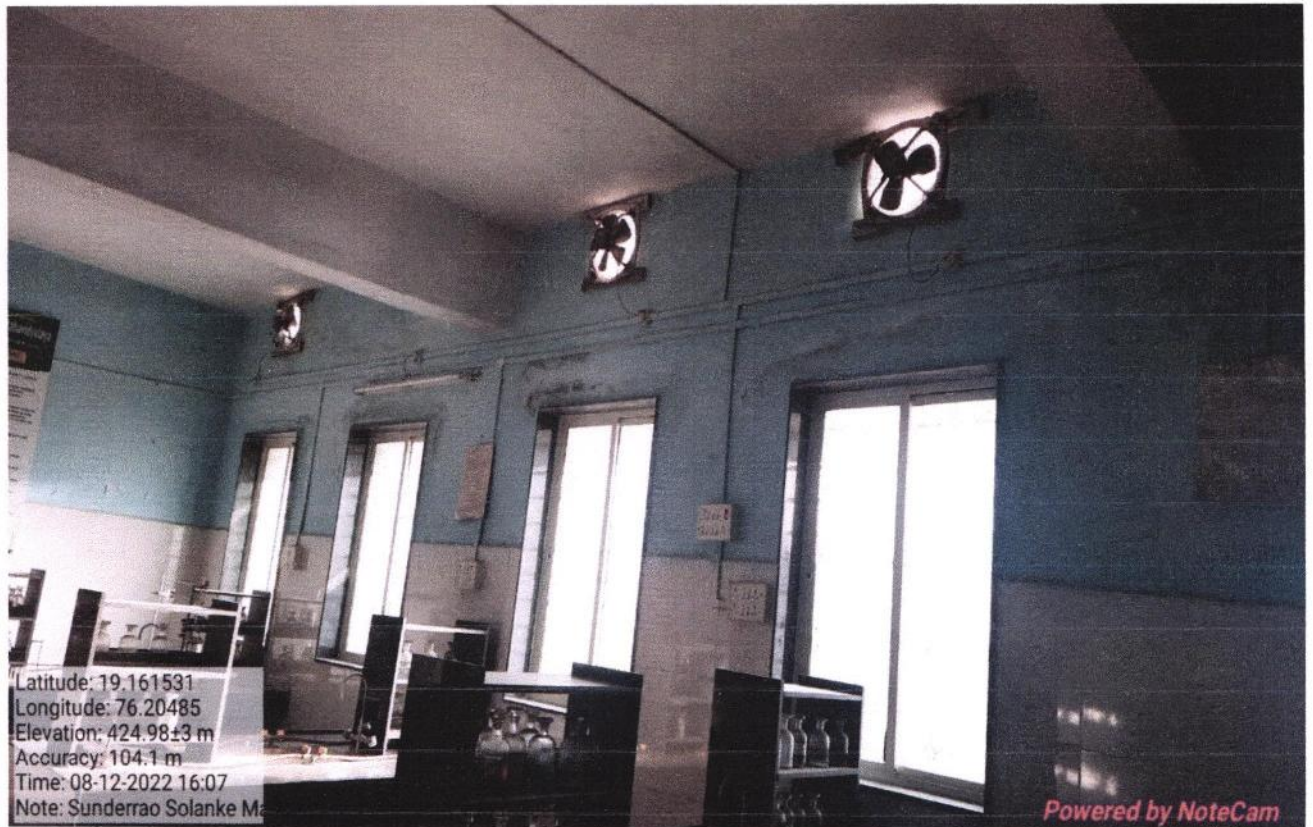
Exit Fans in Chemistry Labs
