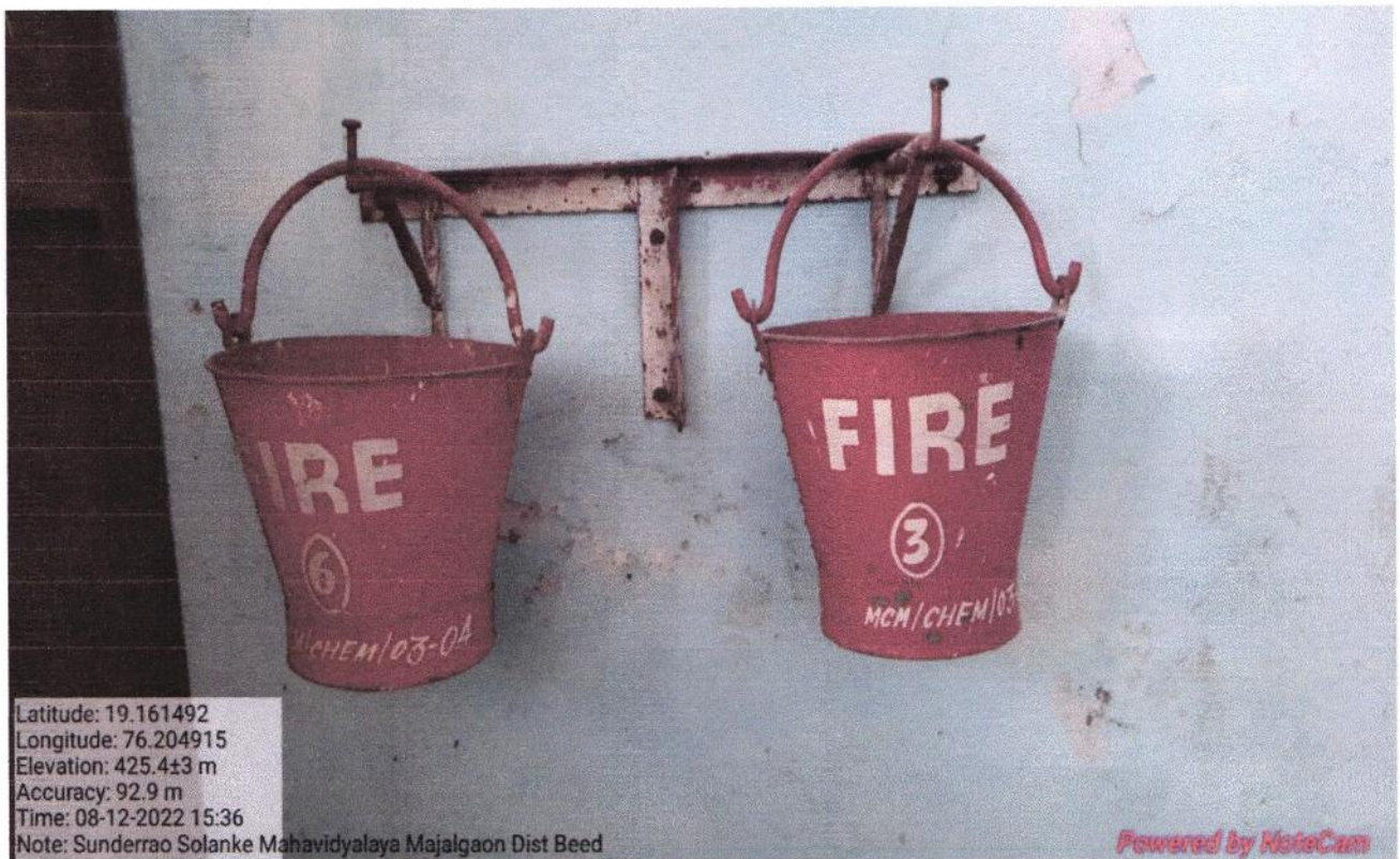
Fire Safety Bucket
