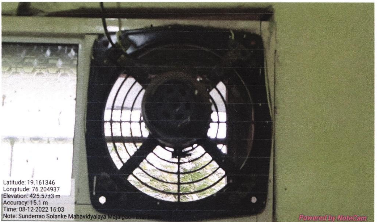
Exit Fans at Wash Room
