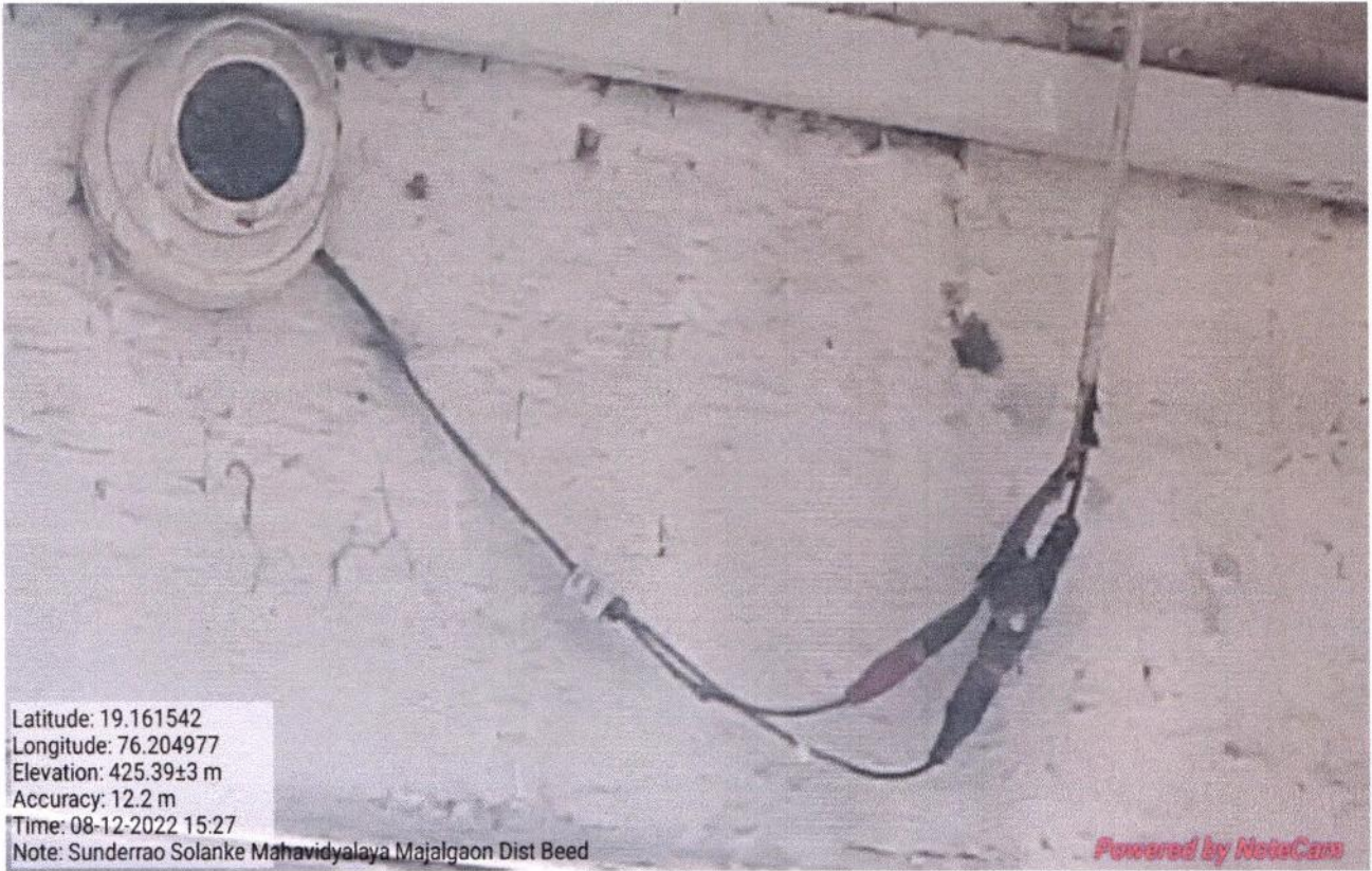
CCTV Camera at Science Building entry Gate& Ladies Common Room
