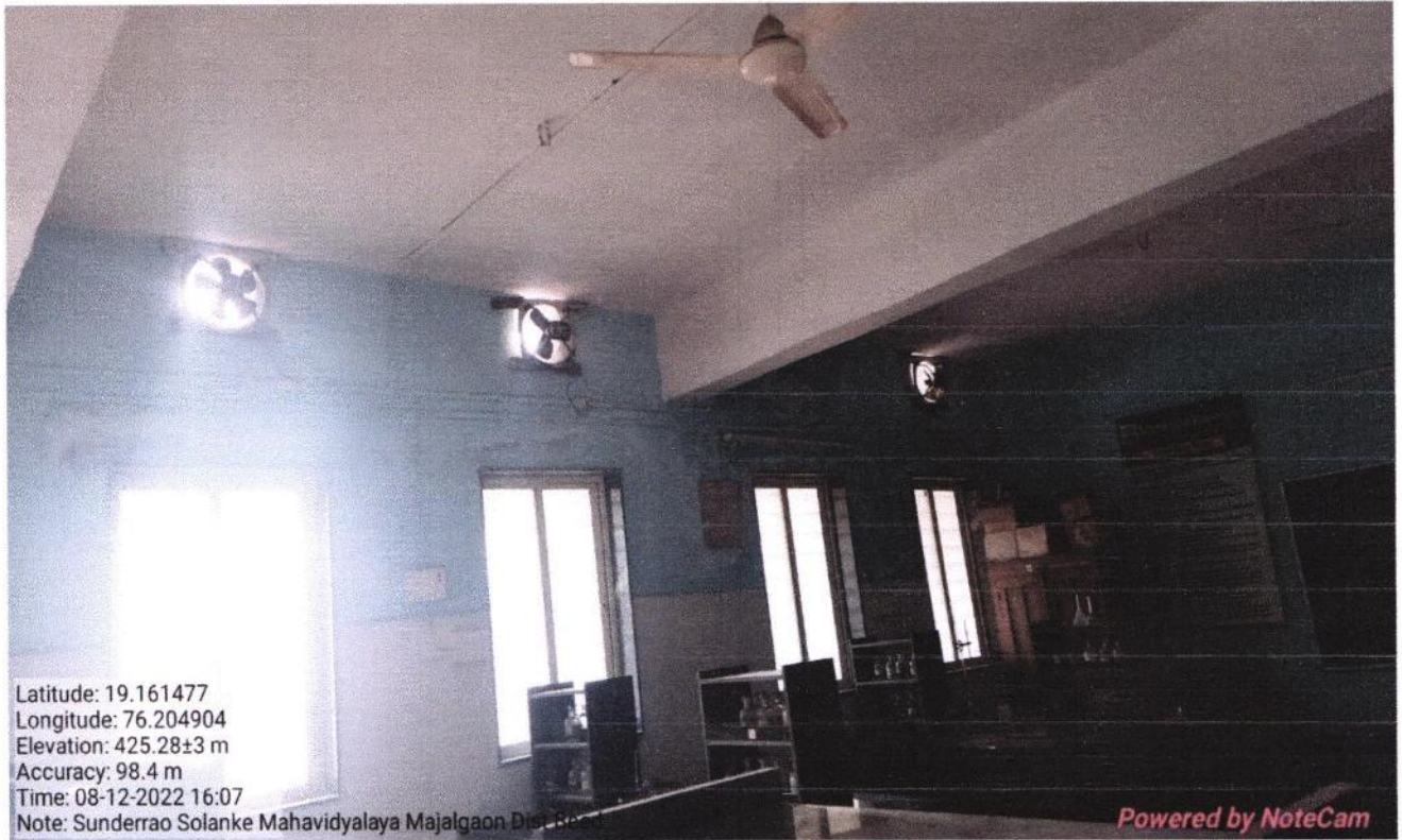
Exit Fans in Chemistry Labs
